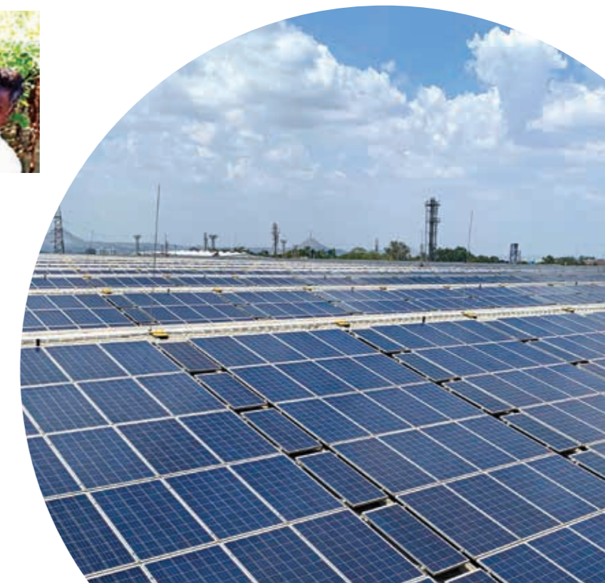
Roof top solar at Nashik plant
